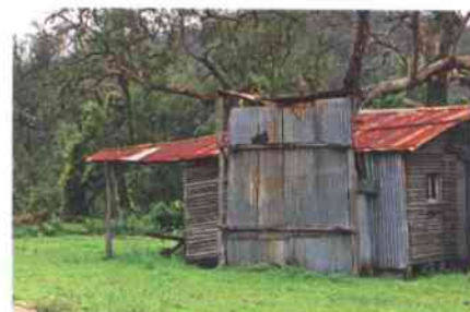
The iron sheets in this old bush hut have rusted.
